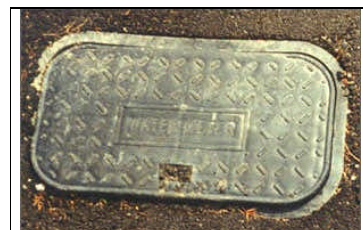
Can't find the water meter? Look for a round or rectangular box lid in metal or black plastic, near the road entrance to your house or flat, labelled 'meter' in raised lettering. Lever it open with a screwdriver. (Meter types vary - study group facilitator has pictures of several others, for reference)
