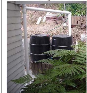
NZ-made rain-water storage barrels by RainSaver Systems of Nelson 03 548 7044 www.rainsaver.co.nz are fed by the spouting. In the best systems a 'first-flush diverter' sends the initial rush of dirty water away from the tank, after which it collects until the tank is full, then overflows additional rain to storm drains.
